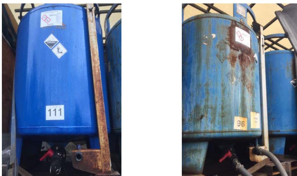
Figure 3: Sodium hypochlorite bulk tank (left) and ferric sulphate bulk tank (right) with labelling before the event
