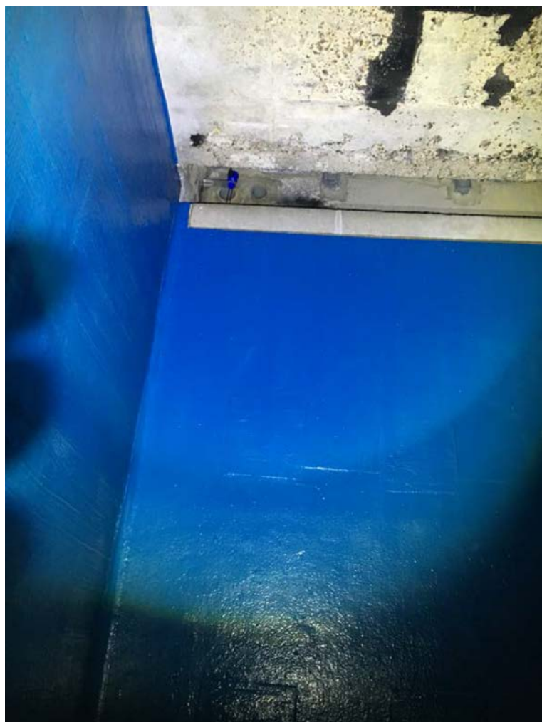
Figure 2: Gap between Weirwood Contact Tank & Backwash Tank
